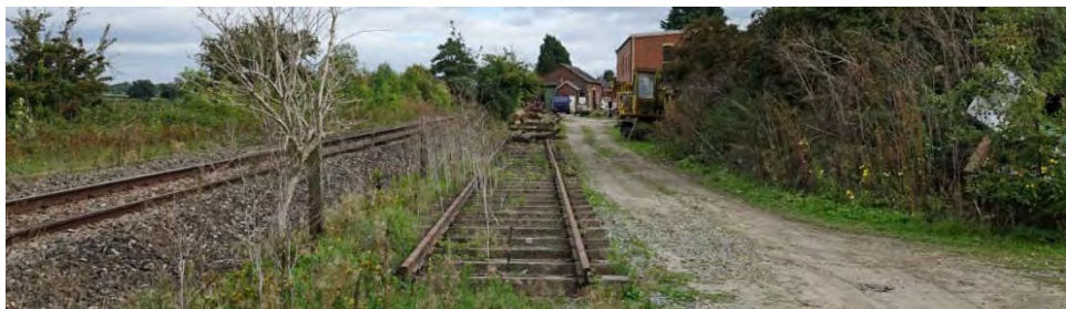
above looking east from the end of the former goods yard with the mainline left, re-laid track and the new loco maintenance shed right beyond the trees which contain the GUV
