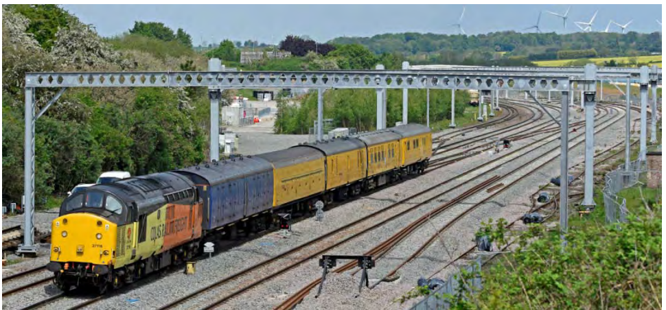
below 37116 t&t DBSO 9702 3Z03 Derby RTC - Tonbridge West Yard approaches Wellingborough underneath the growing forest of OHL masts (12.34) 20 th May 2019 (Colin Pottle)
