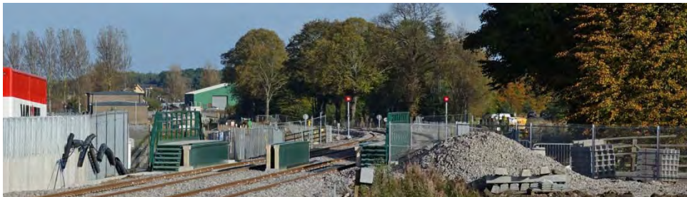
above the former level crossing in front of the beams carrying the double track over the Burn of Mosset, 21 st October 2017
