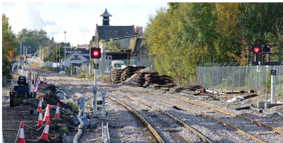
At Elgin work on the platform extensions started in earnest in the summer of 2017 and as the blockade approached new signalling and track appeared along with various infrastructure improvements. Then as the blockade started, around midnight on Friday 7 th October Elgin West signal box was taken out of use. Before then 60075 t&t 60085 had arrived with a ballast working and shunted into the yard. By mid morning on the Sunday the orange army had made short work of demolishing the signal box and the level crossing, with the debris being loaded onto road trucks. Track had been lifted east of the station and the trackbed for the extended loop was excavated from the station to the level crossing to connect to that already laid as seen in the Jul / Aug 2017 issue. As the week progressed infrastructure was laid and the signals tested. All track, apart from the short stretch in platform 2, was replaced. Friday the 13 th saw 66565 arrive with a ballast train and Tamper DR 73904. (see photo of this elsewhere).
